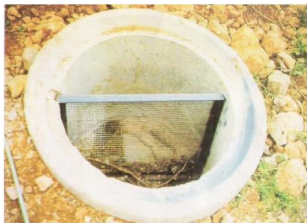
Figure 2-16: Screening manhole in PARC system.
